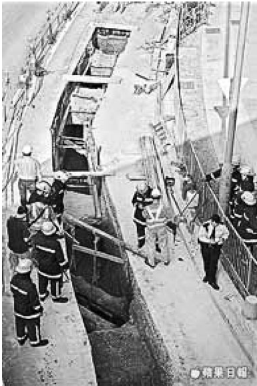
Figure 2.5 - Electrical Explosion in Excavating Open Trench
